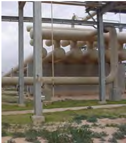
Slug catcher at the Hannibal terminal, U.K.
