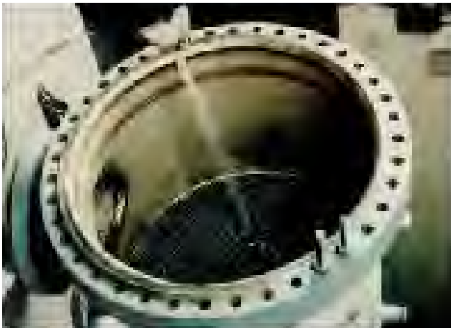
Under-performing, 324 tube, heat exchanger
